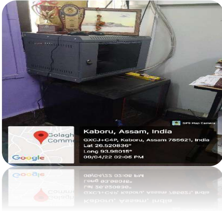
Server In Principal's Chamber
