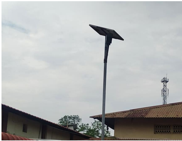
A Solar Panel
