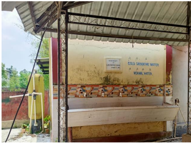
Water filter and drinking water tank with taps
