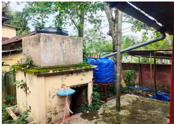
Rain Water Harvesting & storage
