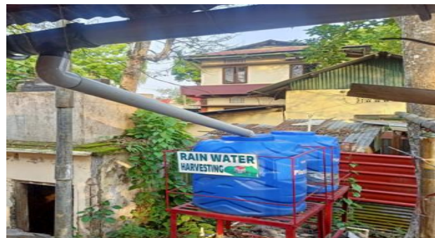
Rain Water Harvesting
